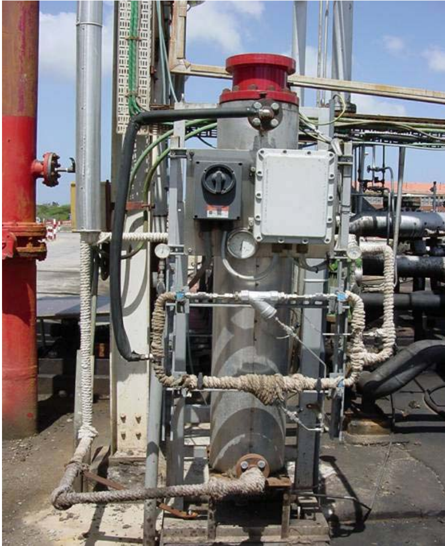
Crude Fast Loop Heater
